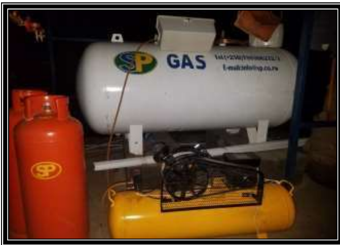
SP LPG INSTALLATION RWANDA
