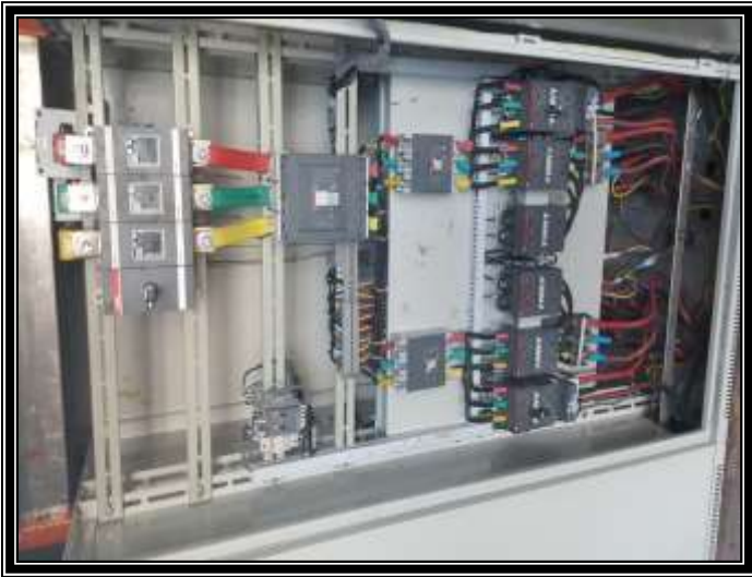
LEREXCOM DEPOT ELECTRICAL MATADI
