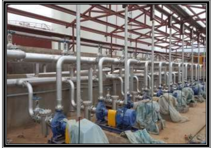
MPIKA PUMP INSTALLATION ZAMBIA
