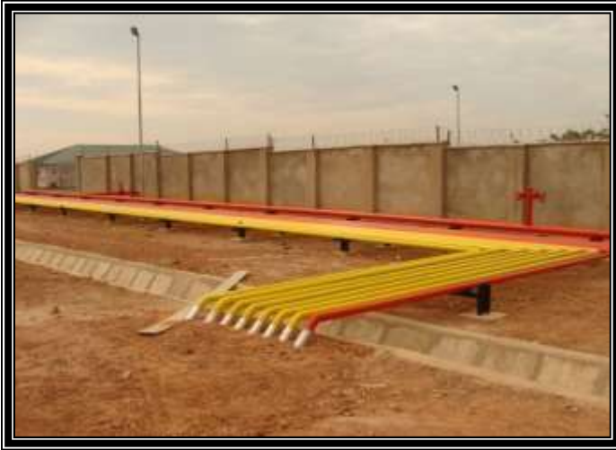
MPIKA DEPOT FIRE PIPE LINES ZAMBIA
