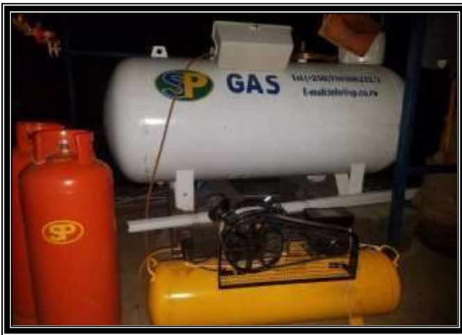
SP LPG INSTALLATION RWANDA
