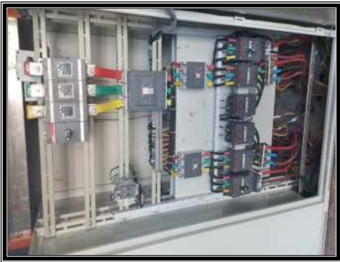
LEREXCOM DEPOT ELECTRICAL MATADI
