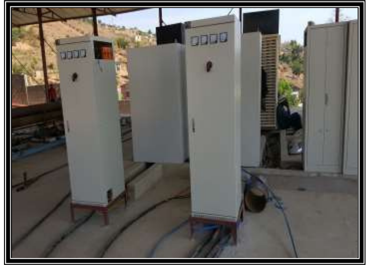
LEREXCOM ELECTRICAL MATADI CONGO
