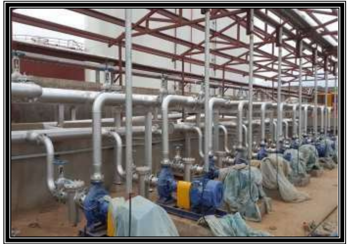
MPIKA PUMP INSTALLATION ZAMBIA
